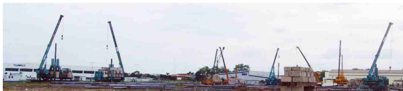
海防5台静力压桩机施工 Construction scene of 5 static pile drivers in Haiphong
