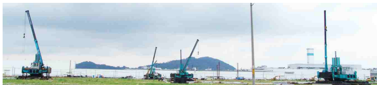
广东南海8台静力压桩机同时施工 Simultaneous construction scene of 8 static pile drivers in Nanhai, Guangdong
