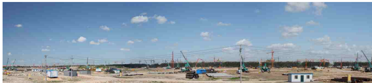
大庆油田多台静力压桩机施工现场 Construction scene of multiple static pile drivers in Daqing Oilfield
